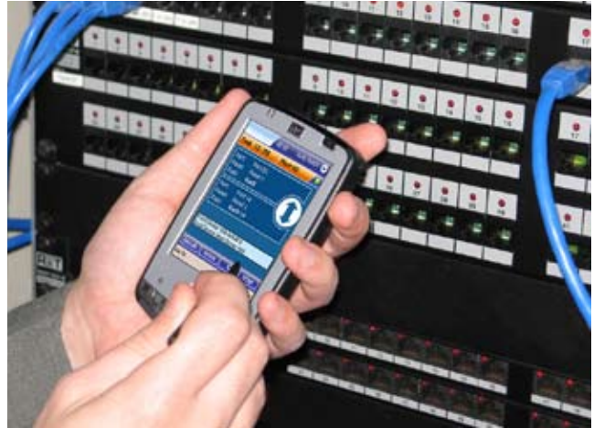
Hand-held devices that come with some IIMS are vital tools for IT professionals and infrastructure engineers on the move, bringing advanced management capabilities out into the field.
